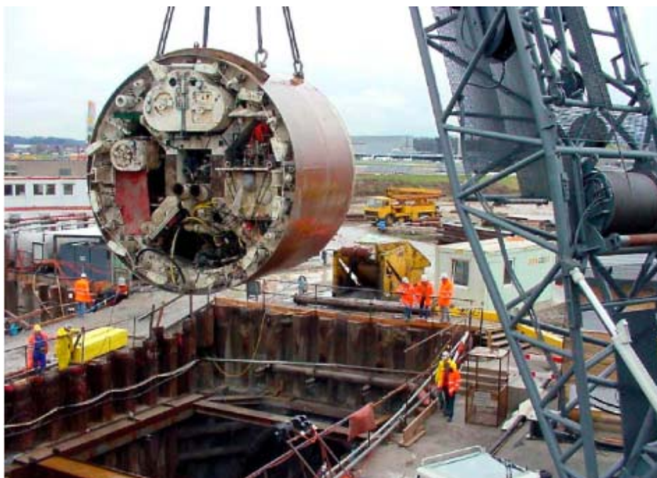
Figure 32: Installation of a hydro shield TBM for tunneling under Zurich airport (Amberg archive)
